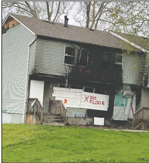
Olive Park Village Unit A has extensive fire damage and will be demolished soon in accordance with a Circuit Court judgement.
